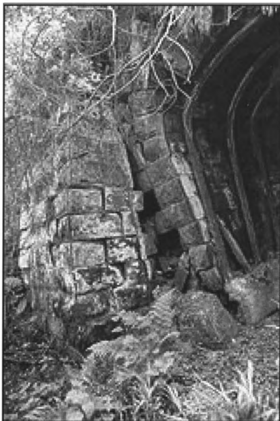
Figure 21: the north portal of Deepgrove Tunnel on the verge of collapse. In 2008 six feet of the roof collapsed
