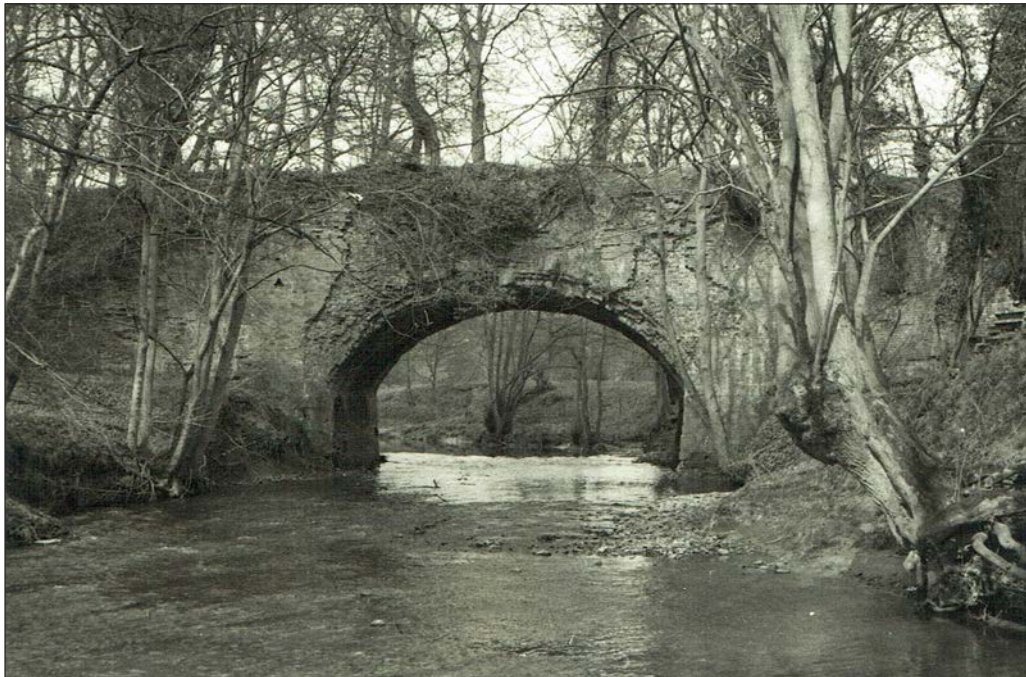
The aqueduct over the River Rea on part of the canal which has never been formally abandoned. Photographed in 1964, it has deteriorated since.
