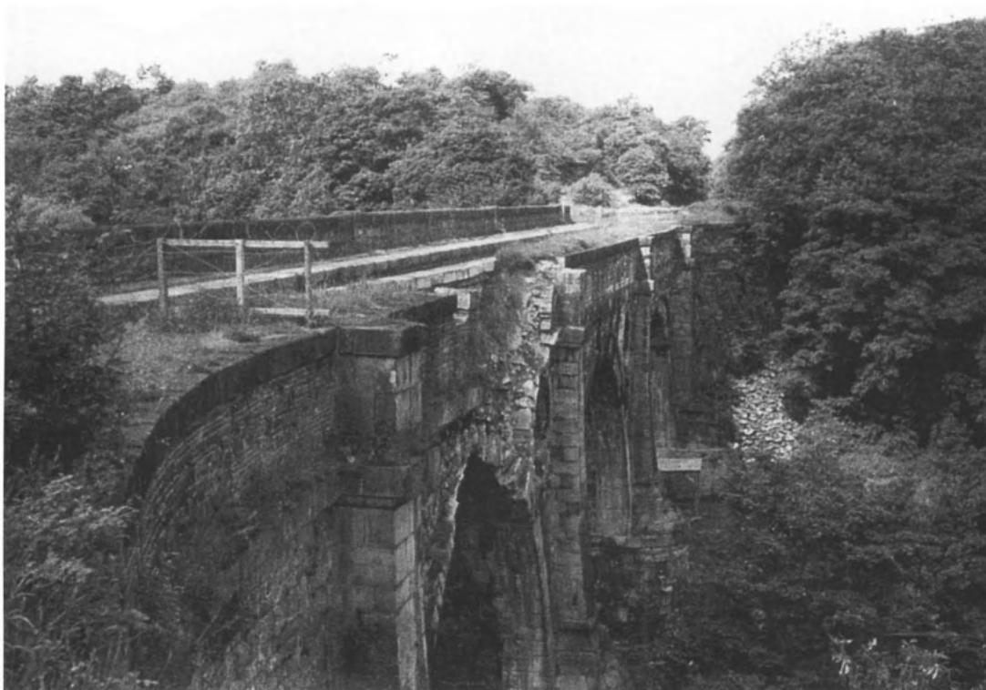
MARPLE AQUEDUCT BREACH 1962
